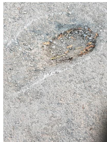
(c) An area marked for attention in Blewbury Road
