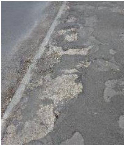
(a) An example along Main Road where a fall occurred
