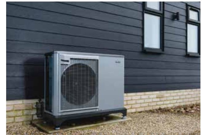
Figure 93: Example of an electric heat pump that is placed to the back of the house, whilst its grey colour fits nicely with the black weatherboarding of the property.
