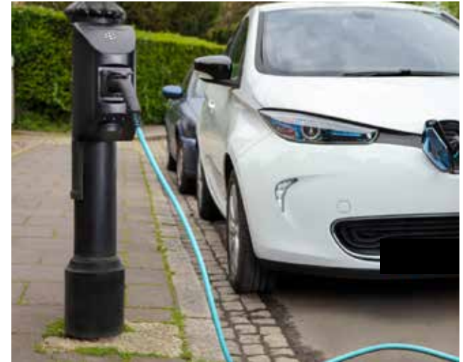
Figure 96: Example of on-street electric vehicle charging points.
