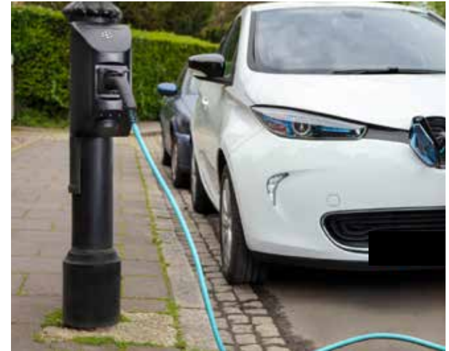
Figure 96: Example of on-street electric vehicle charging points.
